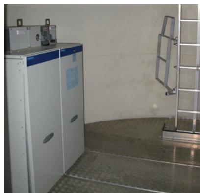
Wind farm application (Denmark)
